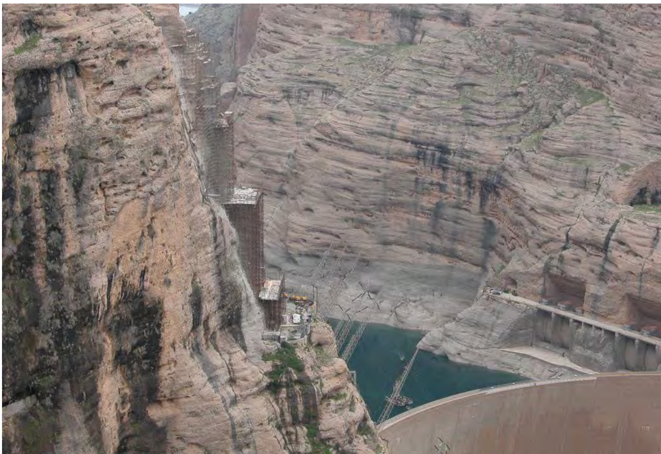
Dez Dam IRAN Contractor: Iran Water Resources Development TPE 02SP permanent anchors according to EN 1537
